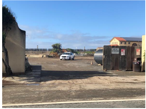
The Sharp Park Pump Station is undergoing an odor control upgrade to make it compatible with any future redevelopment of the 2212 Beach Boulevard site.
