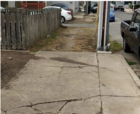
While there is dedicated space for a sidewalk, the quality and safety are inconsistent.
